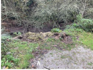
A - Back to the parking area, there are grass clippings but no planting or trees in this area. Grass clippings need to be disposed of off site.
